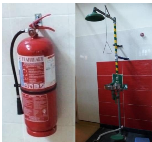
Fire extinguisher, eye wash and safety shower in First Year Laboratories.
