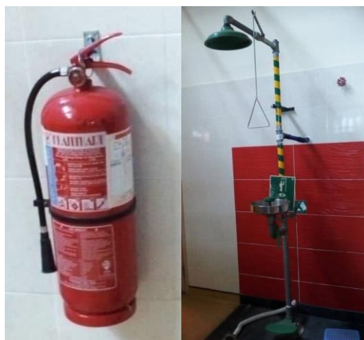
The fire extinguisher, eye wash and safety shower in the Second Year Organic Laboratory
